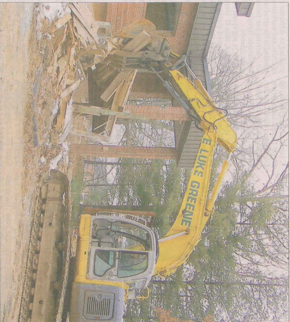
PHOTO PROVIDED A 70,000-pound hydraulic excavator takes down a section of the porch and steps at Blue Ridge Community Health Services in the first step of demolishing an old clinical building in order to build a new facility.
